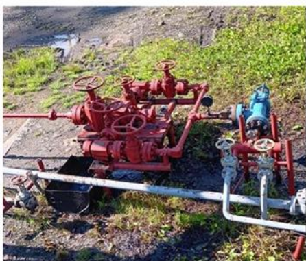
Fig. 6. The existing choke manifold
