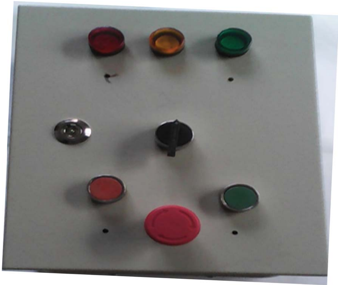
Figure 5 Picture of the DOL starter showing the various push buttons and indicator lights after the completion of the wiring of the main circuit and the control circuit.
