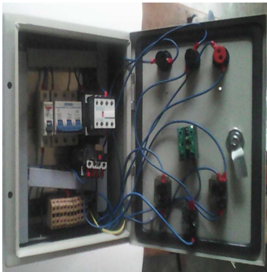
Figure 4 Picture of the DOL starter after the completion of the wiring of the main circuit and the control circuit.
